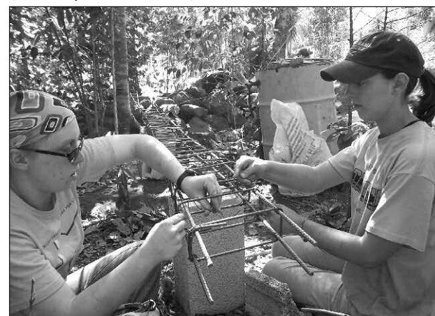
Kristin Alphin, from Azle, Texas, and Jenny Stahl, from Apple Valley, Minn., put together rebar forms used to reinforce the concrete foundations of the homes under construction. (Photo by Beth Wensel)
